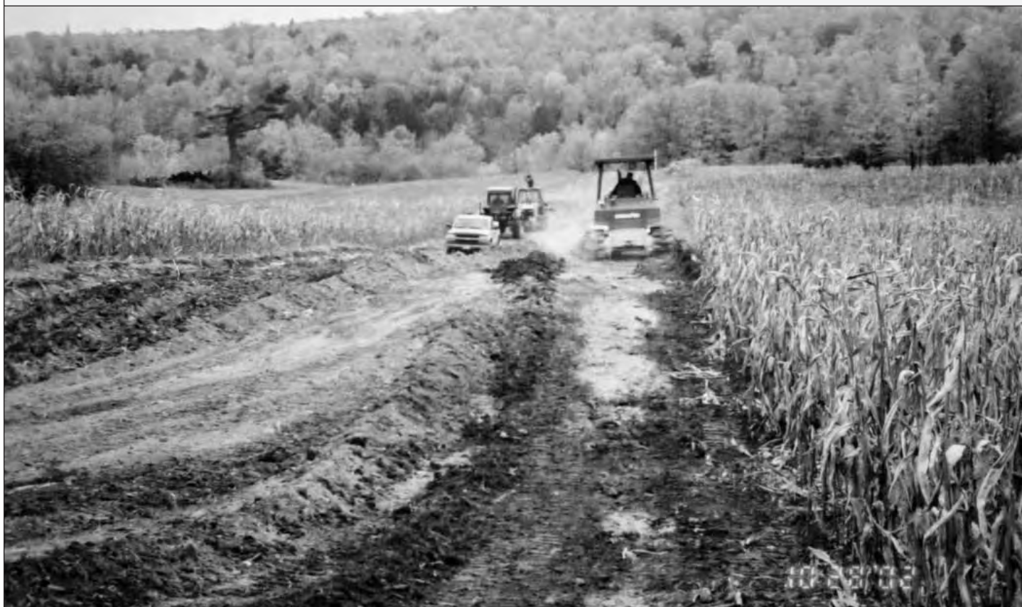
Pipeline construction leaves an ugly path through a cornfield. Photo by John Lacey
