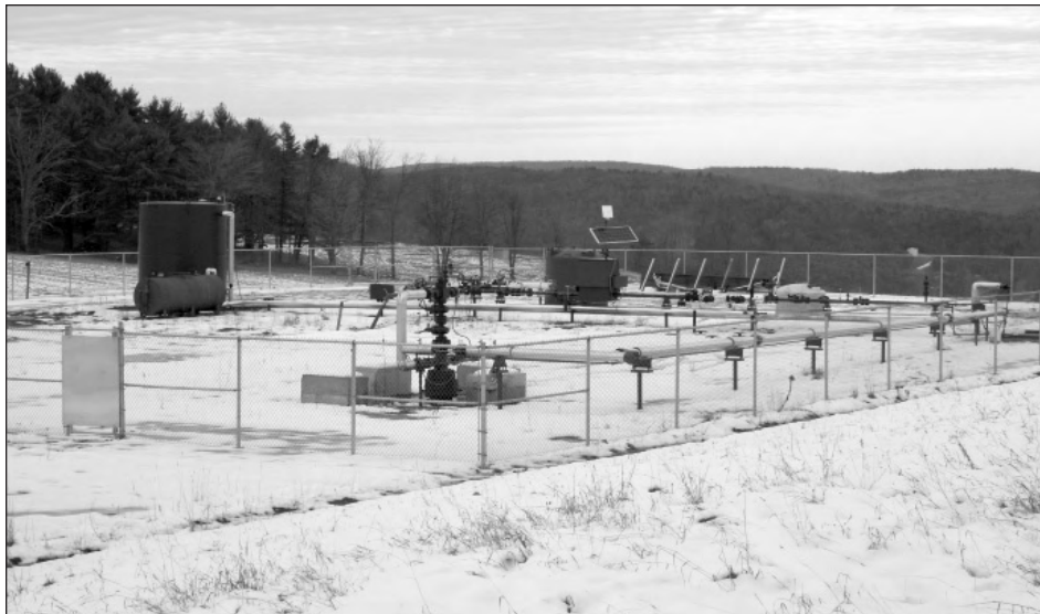
Fortuna Energy Inc. is planning to test the nonproducing Mallula well in Van Etten, New York, as an underground waste disposal site for drilling wastewater. Photo by Sue Smith-Heavenrich
